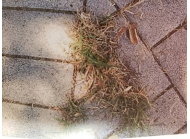
Weed Growth within joints
