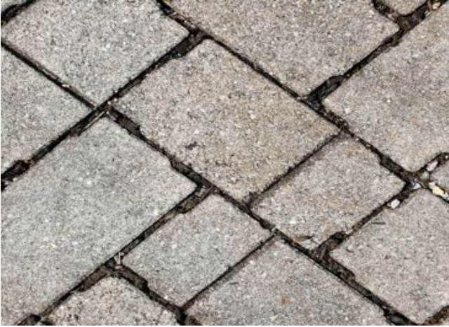
Sediment Crusted Joints
