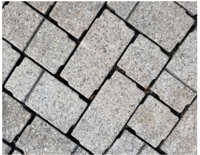
Insufficient joint stone
