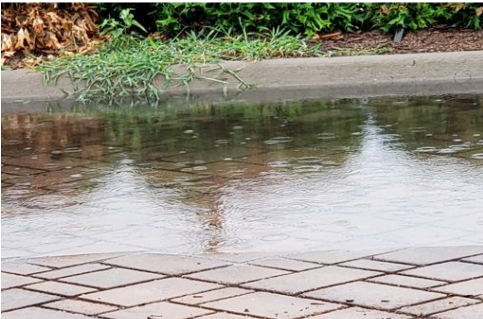
Figure 1 Surface ponding due to sediment build up.
